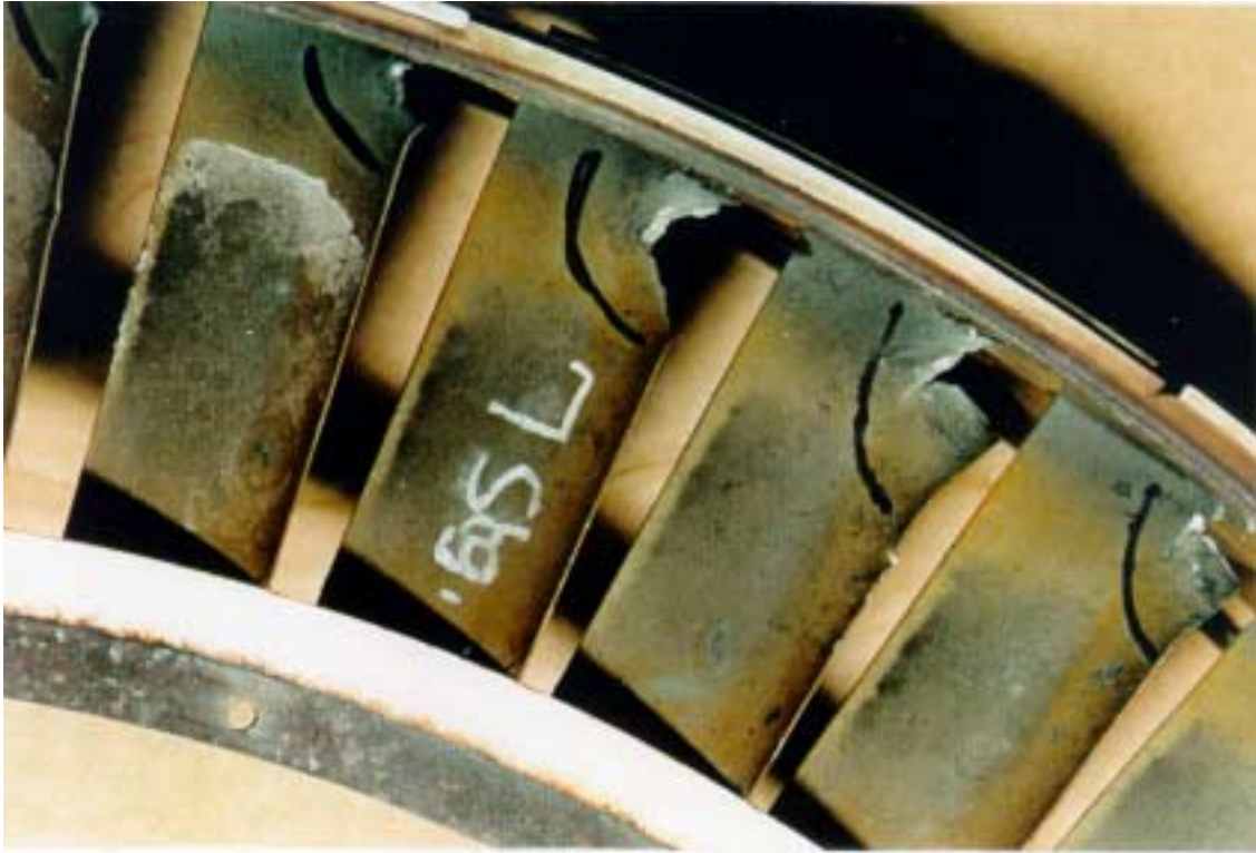
Figure 3. Some of the compressor 7th stage stator trailing edge damages
