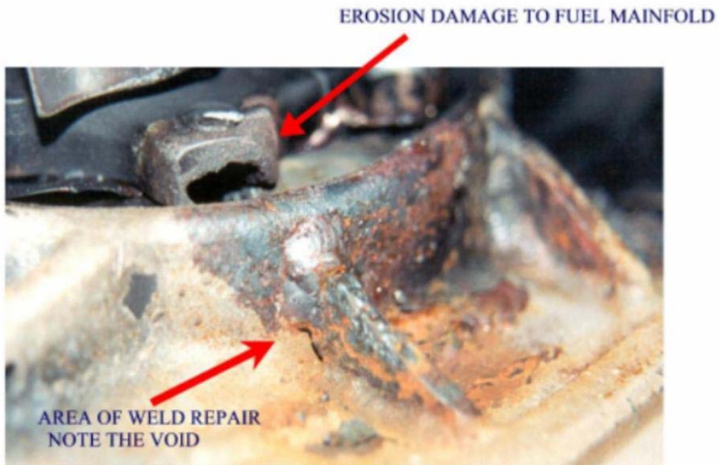
PHOTOGRAPH OF THE INTERIOR OF THE DIFFUSER CASE SHOWING THE P&D VALVE MOUNTING-BOSS& DETAILING THE EROSION DAMAGE TO THE FUEL MANIFOLD AND THE DEFECTIVE WELD REPAIR
